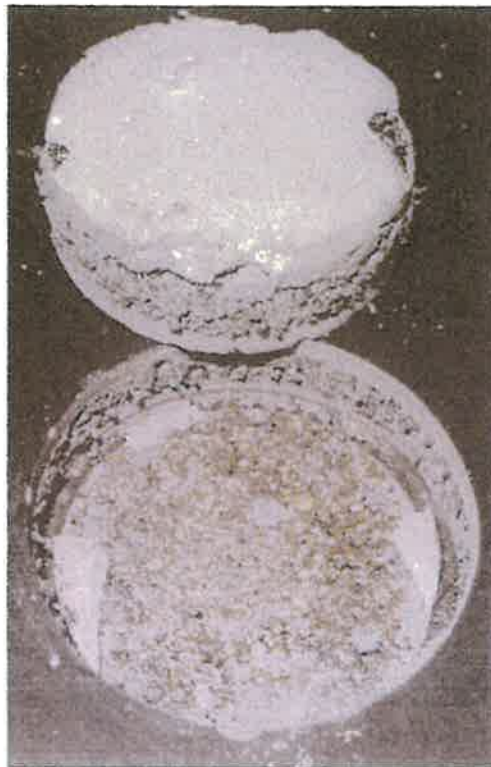
Figure 9. SignaFlor core #4 with moisture mitigation membrane attached to core but not the concrete. Concrete below membrane is damp.
