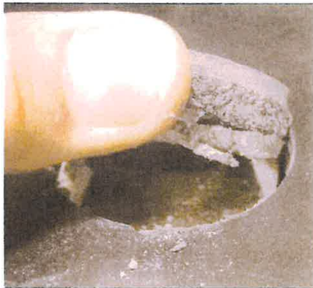
Figure 8. SignaFlor core #4 being removed. Only very weak adhesion to concrete.
