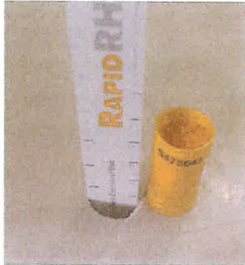
Figure 1. Rapid RH® sensor before insertion into hole drilled in the concrete to measure humidity and temperature in the interior of the concrete slab.
