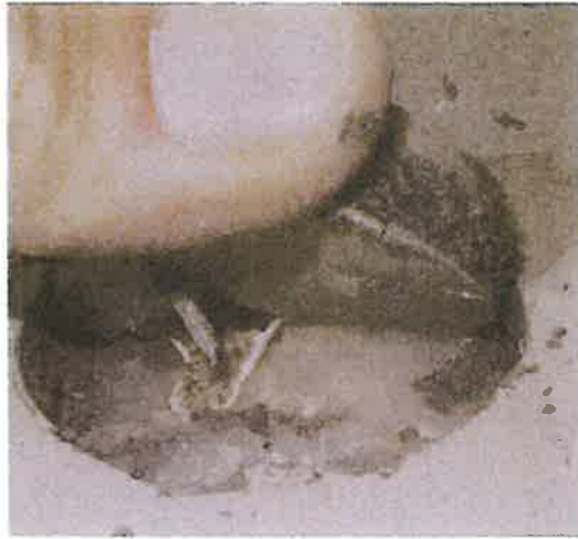
Figure 5. SignaFlor core #2 being removed. The moisture mitigation membrane was firmly attached to the concrete slab. Cohesive failure can be seen within the SignaFlor layers.
