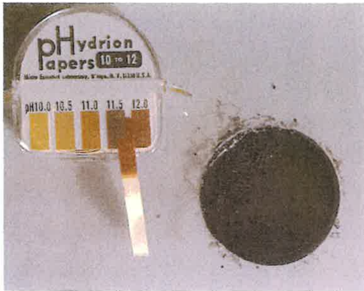
Figure 7. SignaFlor core #3 cavity with highly alkaline water, pH = 11.5 - 12.
