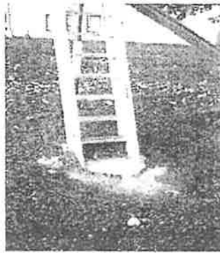
Exposed concrete footing
